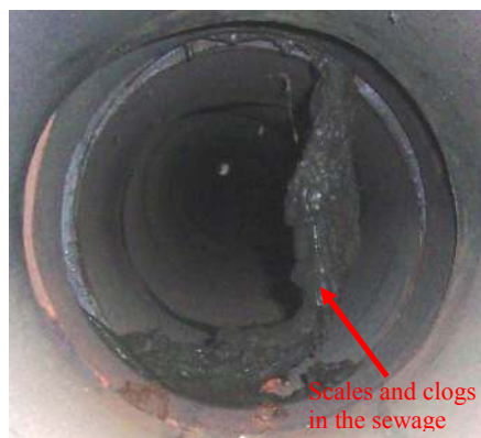
Fig.1 Sewage Pipe with Clogs and Scales
