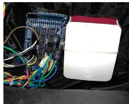
Fig 12. The view of the front compartment of the bag where the systems and the batteries are integrated for controlling the sensors and acquiring the data from the bag.
