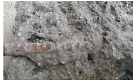
FIGURE 10: Snapshot of plain concrete specimens with corroded rebar.
