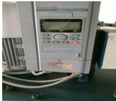
Figure 1: Variable Frequency Drive
