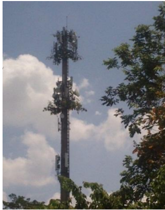
Figure 1. Base Station Tower.
