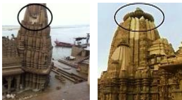
FIGURE 4. Lightning Damages (a) Rathneswar Mahadeshwar Temple and (b) Jagadambika Temple in 2016 and 2015 respectively
