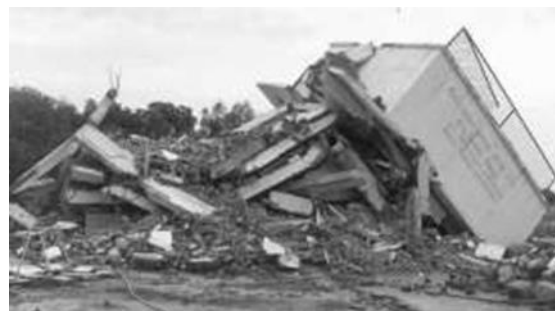
(b) Collapsed weak frame staging
